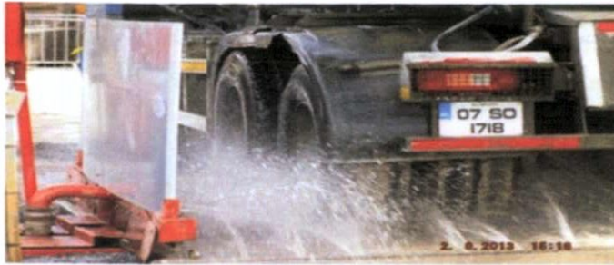
Figure 8 - Typical Wheel Washing Facility
