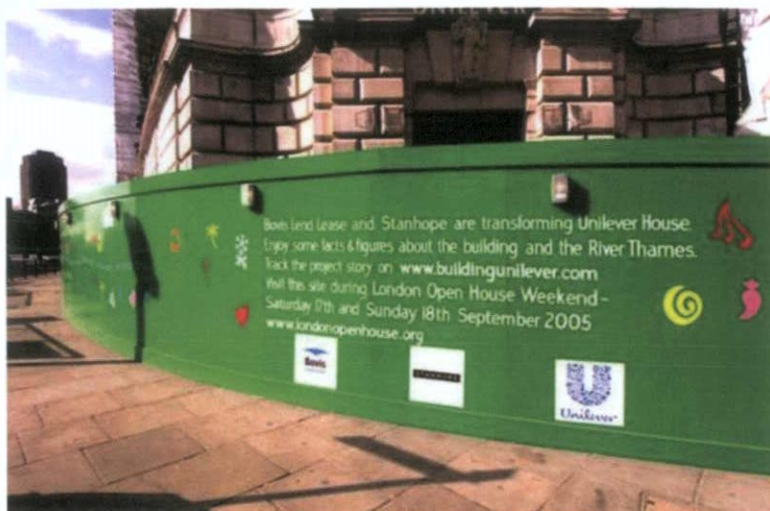
Figure 5 – Typical pavement hoarding with street lighting
