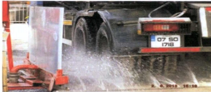
Figure 9 – Typical Wheel Washing Facility
